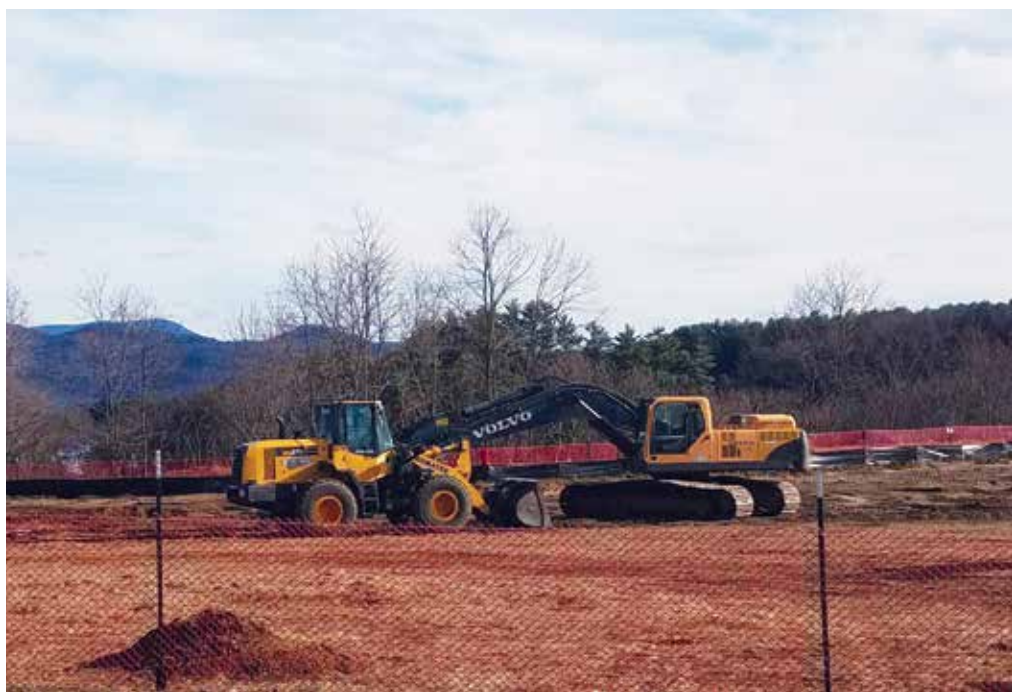
Site work is underway at the location of the Margaret Pratt Community assisted living complex in Bradford.
